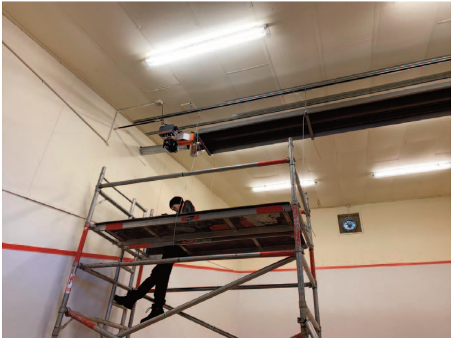
The infamous court 2 replacement heater
